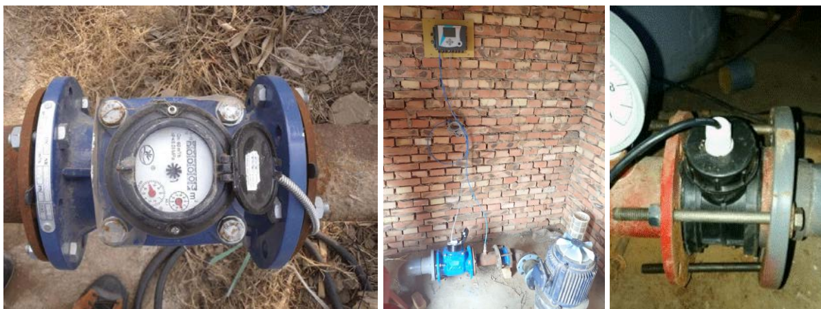
Figure 48: The Hengze meter (left), the Itron meter with transmission unit Watermind on the wall (middle) and the Haisen meter (right).
