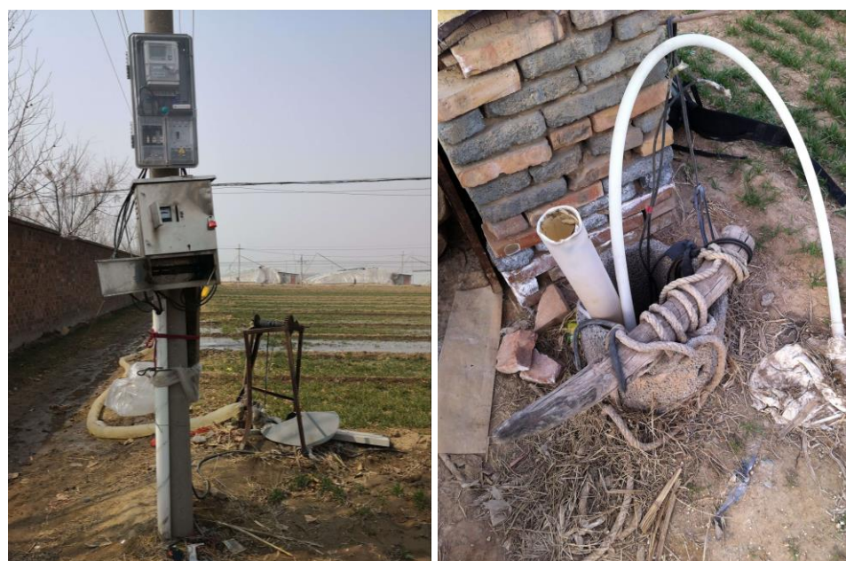
Figure 47: Typical irrigation wells and different meters installed in Guantao County.
