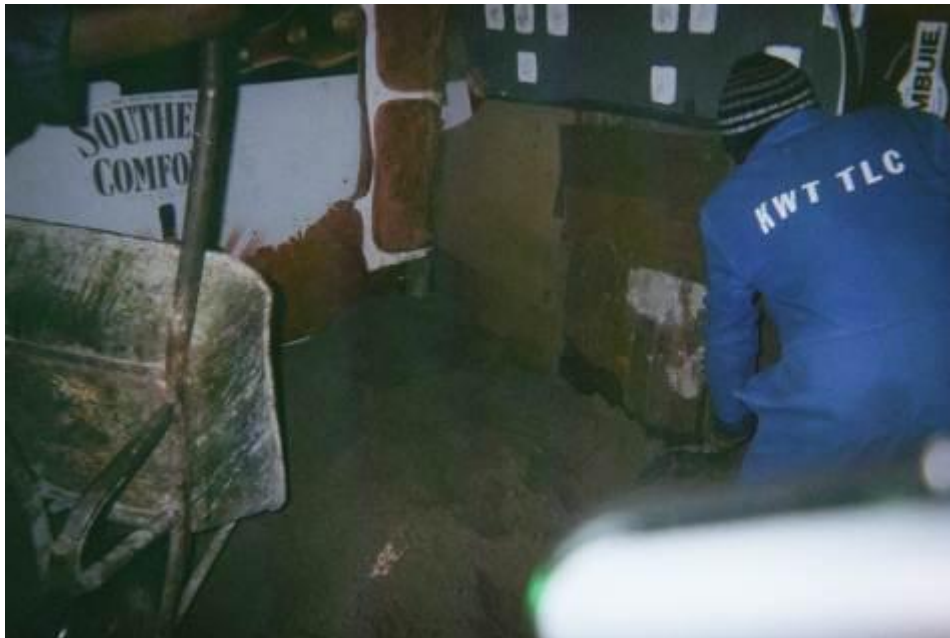
Picture 16: “ They are putting in sand with a wheelbarrow and they are leveling the sand ” (Flooding observer, 16.6.2011)
