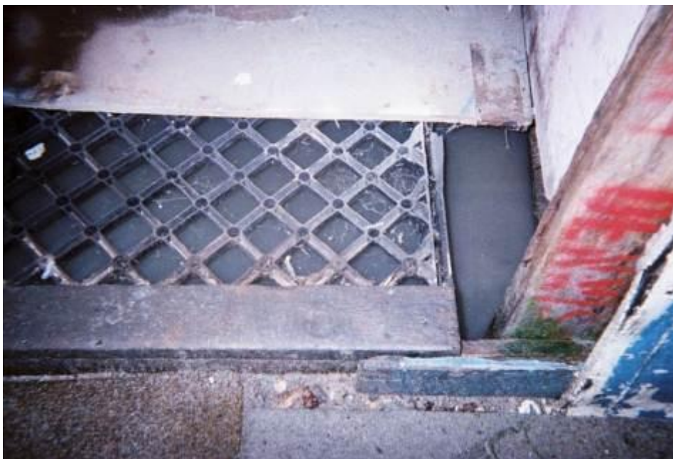
Picture 14: Illustrates the floor in a shack where there is constant water under the floor of this shack, and the person living here just covers it with ceiling boards. She has been living here for 6 years. 14.07.2010
