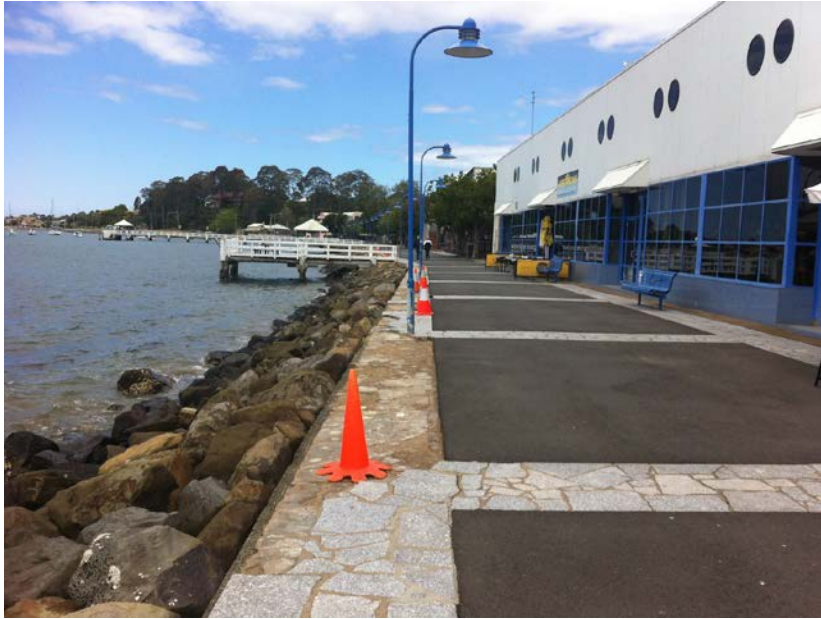
Image: Damage of sea wall in Batemans Bay CBD from coastal inundation (2012) - photo Barbara Norman
