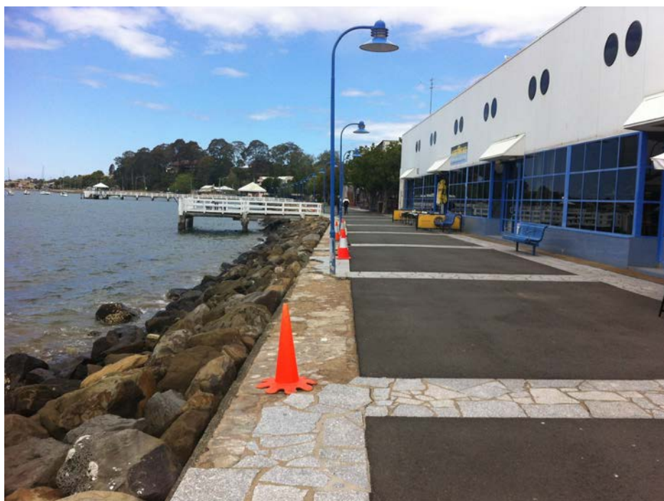
Figure 5. Damage of sea wall in Batemans Bay CBD from coastal inundation (2012) - photo Barbara Norman
