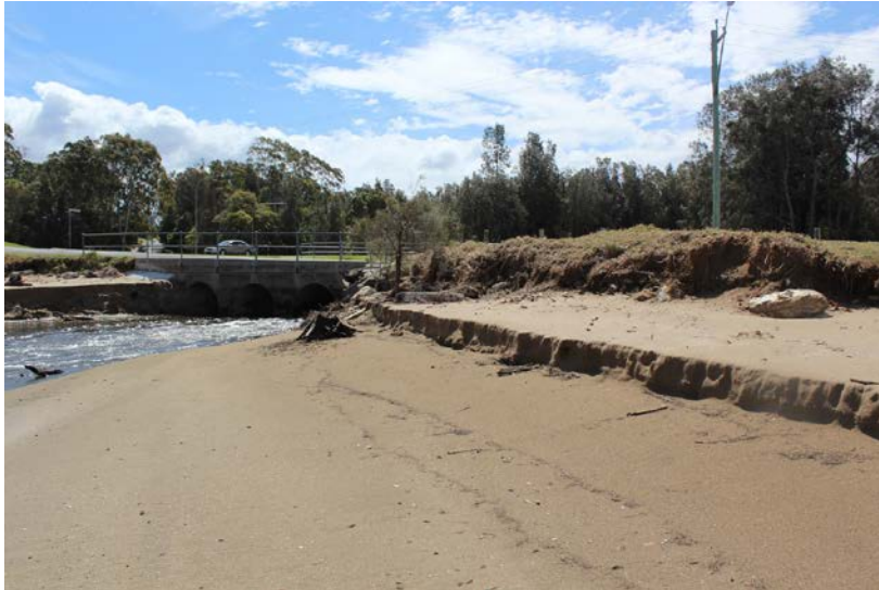
Image: Visible bank erosion near McLeod Street Bridge, Surfside, Batemans Bay (12 October 2012) - photo Kerrylee Rogers
