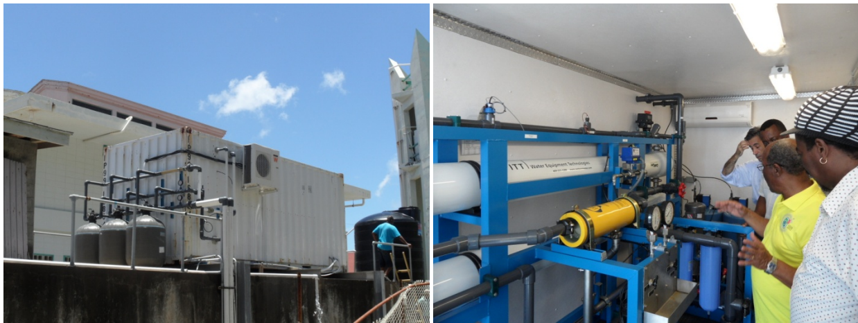
Figure 3: Exterior and interior view of the containerized SWRO plant installed in Bequia
