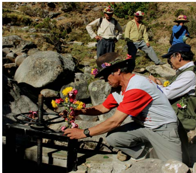
Photo No. 3: Launch of the rehabilitation of a mamanteo system in Huamantanga
