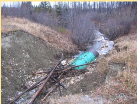
Figure 17. Example of soil erosion at wetland crossing
