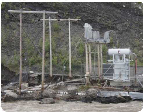
Figure CS1.1 The flood-damaged Barrier 32S substation, June 2013 5
