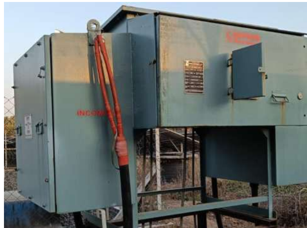
FIGURE 16. The check meter.
