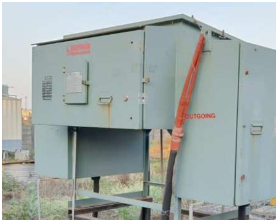
FIGURE 15. The main meter.
