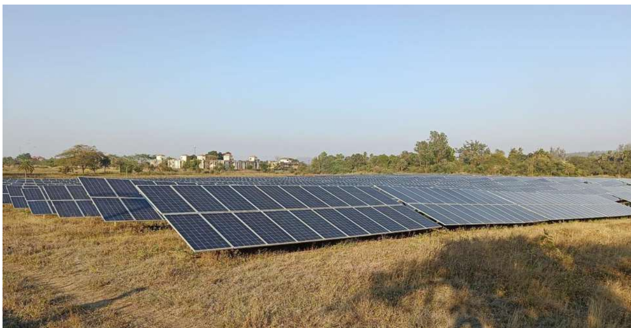
FIGURE 12. The Adani Solar plant at Dapchari village in Palghar district, Maharashtra.
