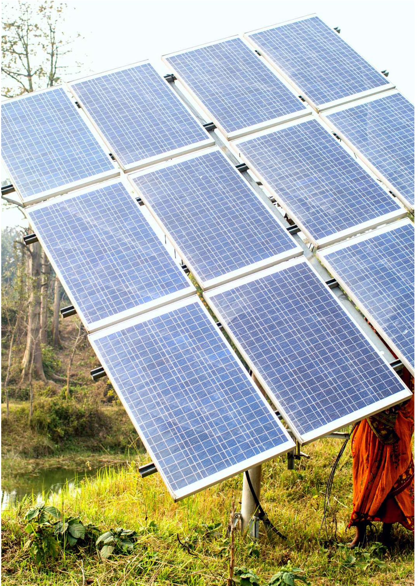
A solar panel installed at Vasedwa Village, Katakariya Municipality, Rautahat District of Nepal. photo: IWMI Nepal.
