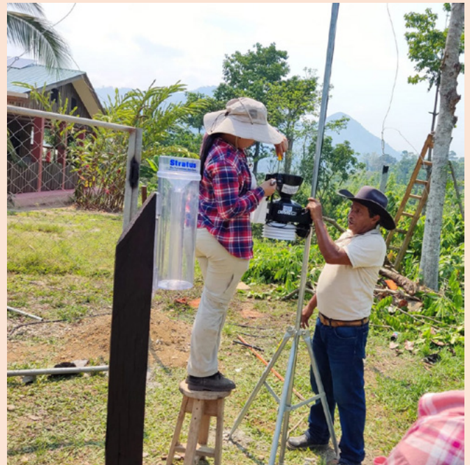
Installation of an automated weather station in Honduras. © FUPNAPIB
