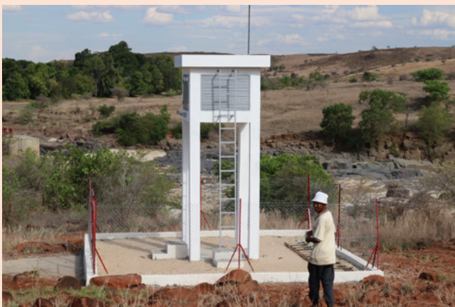
Installation of a weather station in Migodo, Municipality of Ankilizato, District of Mahabo © MEDAIR 2022
